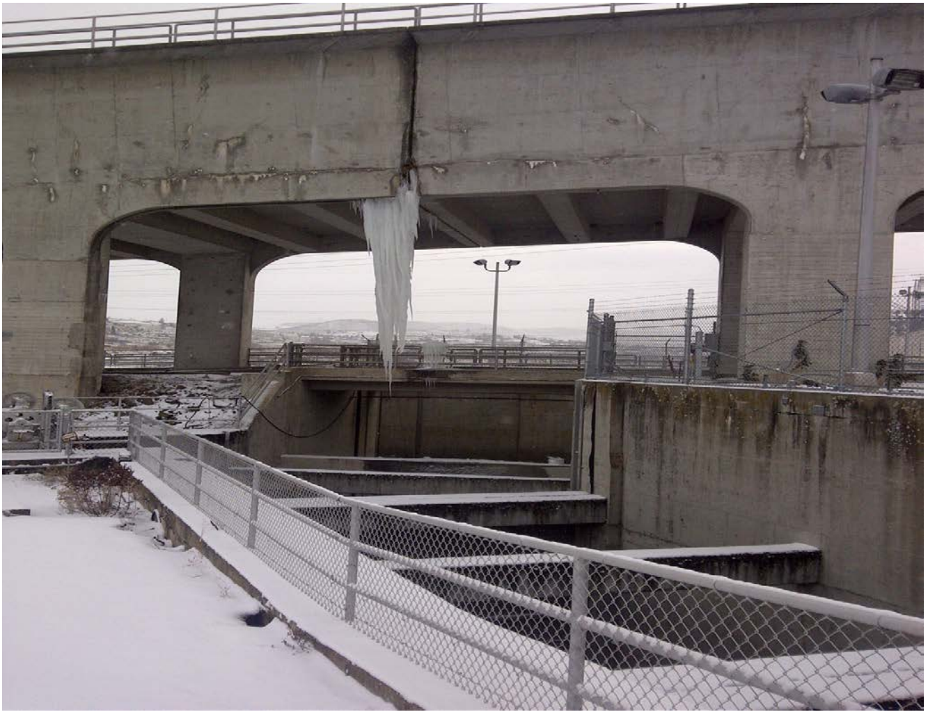
New ice climbing feature forming under east fishladder. Small leak in expansion joint which normally seals as air temperature increases.
